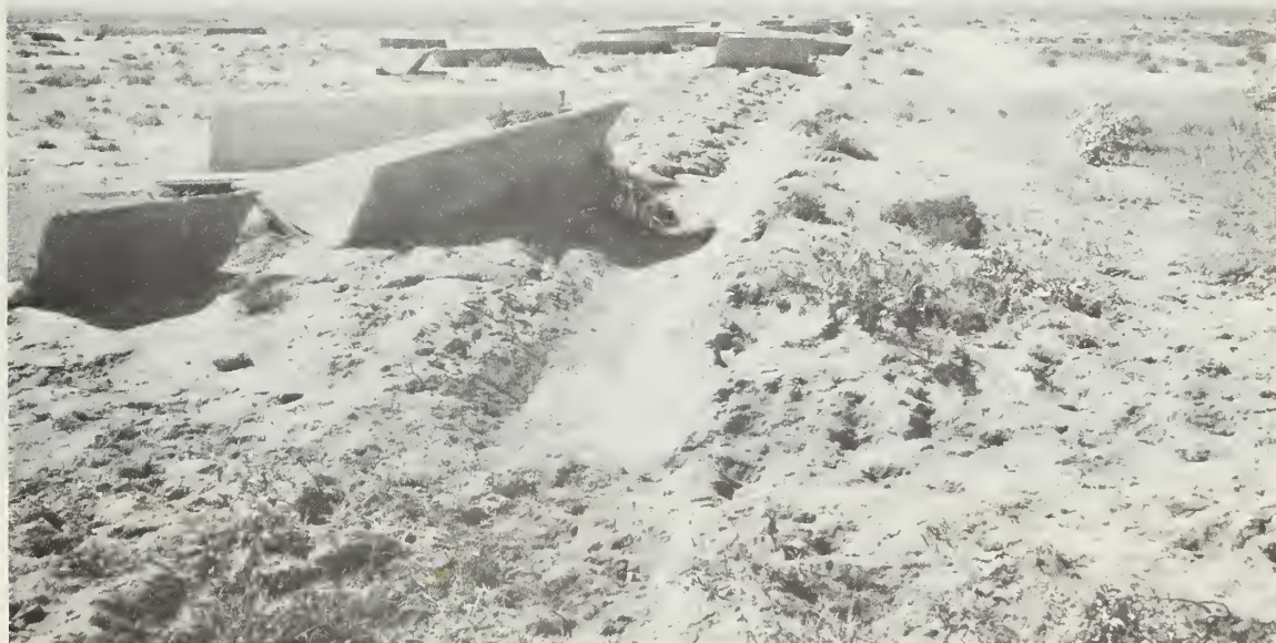
Floodwater damage from flood of August 1966 to irrigation systems in the Wild Horse farming area.
